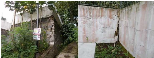
Fig. 7 Cracked building conditions in the research area
