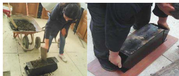
Fig. 2 Placing the concrete inside the mold (left); process to demould the concrete blocks (right).
