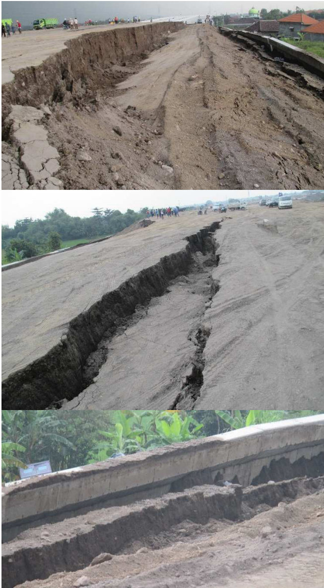
Fig. 1 Landslides reduced the embankment elevation to 3.5 meters and damaged the existing retaining wall due to landslides.
