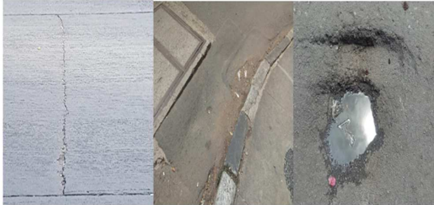
Fig. 5 Identification of Road Damage on Flexible and Rigid Pavement
