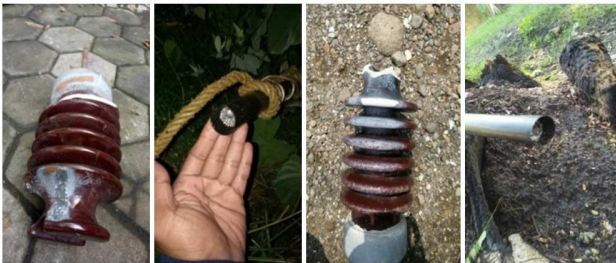
Fig. 1 AAAC-S burn-down and burning a trace on the insulator
